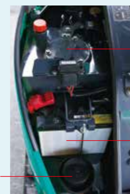
Hydraulic tank Battery
