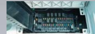
Easy-access fuse box More finely differentiated fuses make it easier to locate malfunctions.
